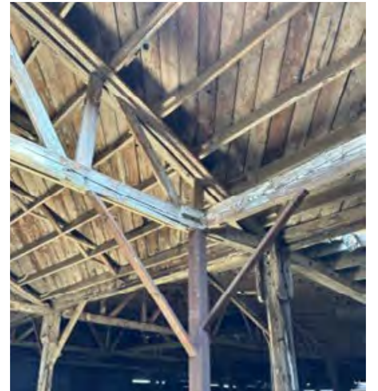
27. Bottom chord failure at truss member with shoring.
