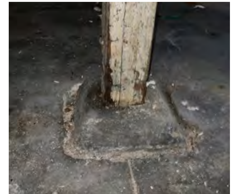
21. Existing concrete column base elevated above concrete slab in several locations.
