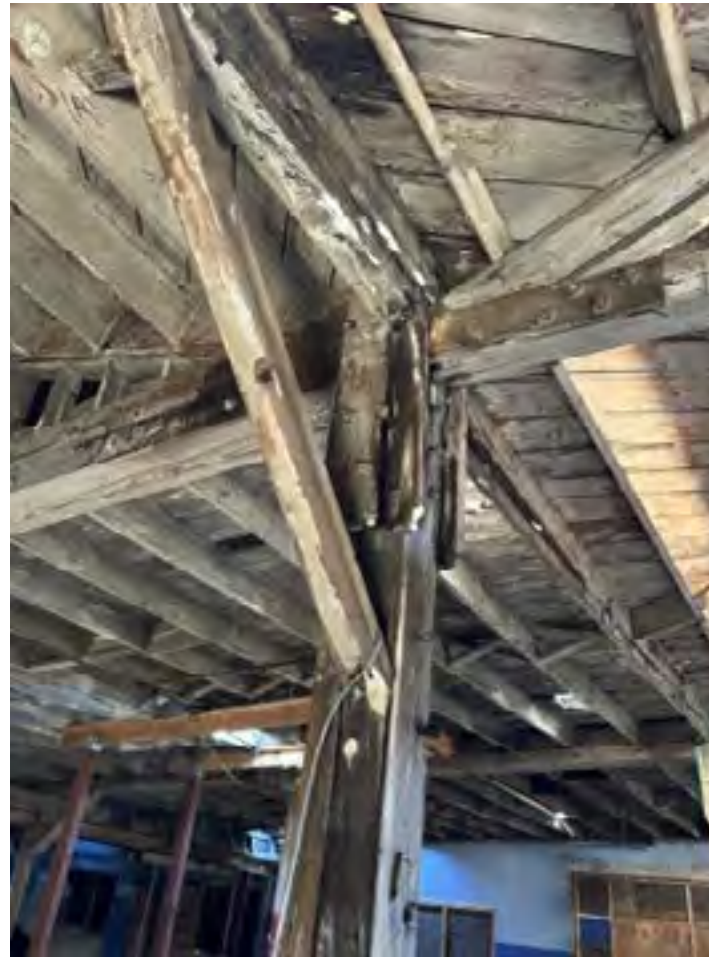
23. Failed connection at interior timber column.
