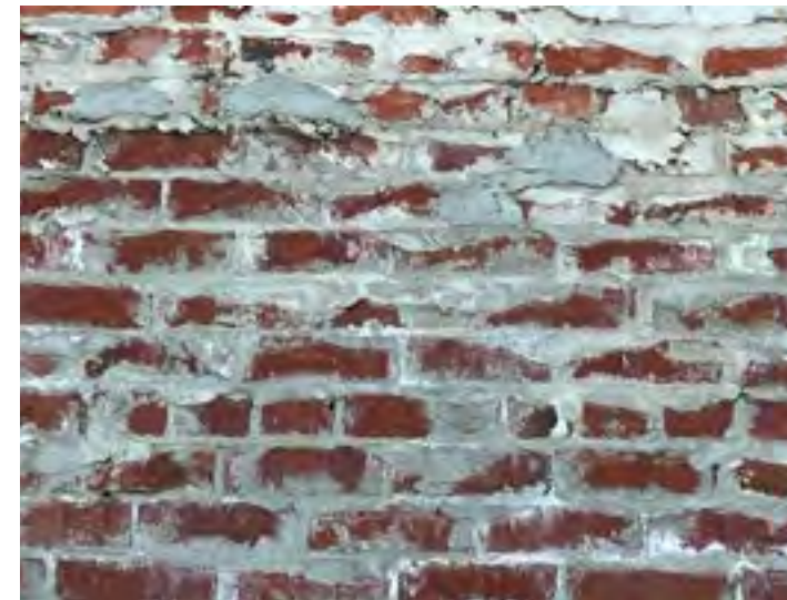
2. Example of east facade brick condition.
