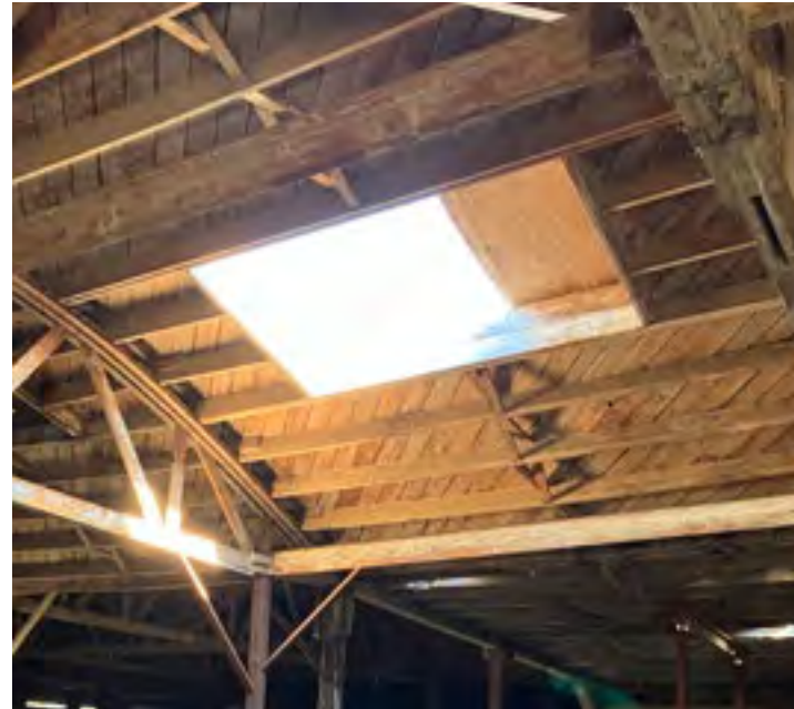
11. Some previously demolished skylight openings have been left uncovered.
