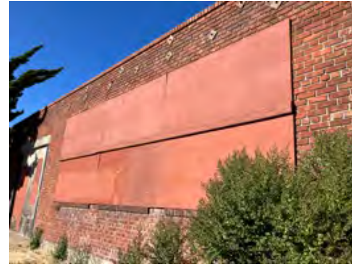
1. Example of west facade brick condition and boarded window openings.
