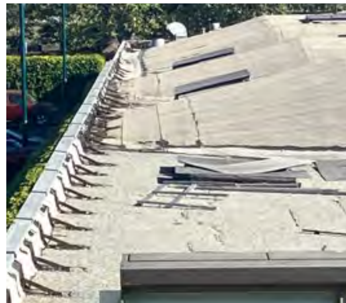
14. View of roof condition from the north. Generally, demolished skylights are covered. Some roof bracket supports are missing.
