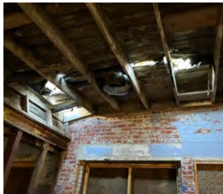
12. Roof deterioration at low point.
