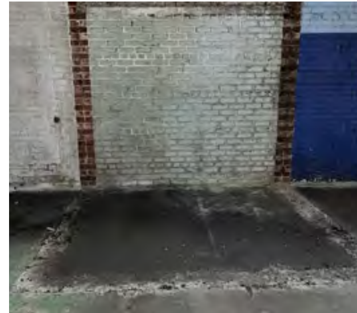
18. Previously demolished interior walls leave existing concrete slab damaged.
