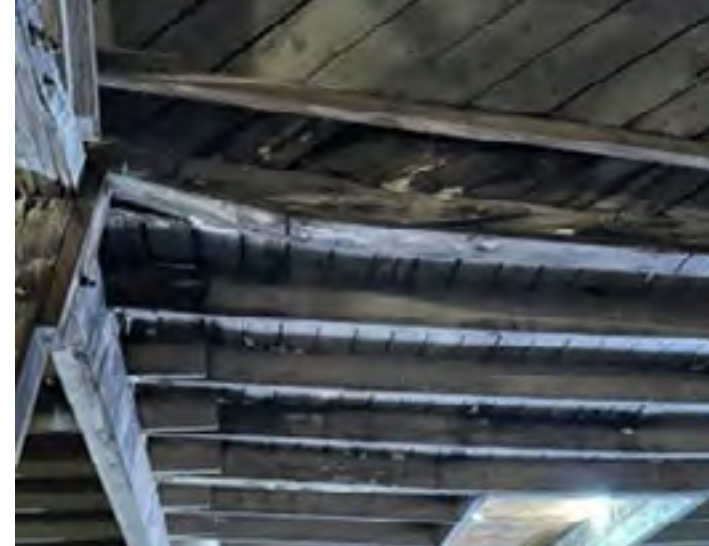
24. Overstressed joint causing failure.
