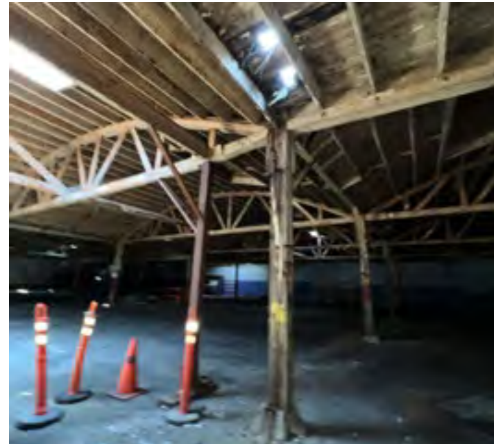
13. Roof deterioration requires shoring in some locations.
