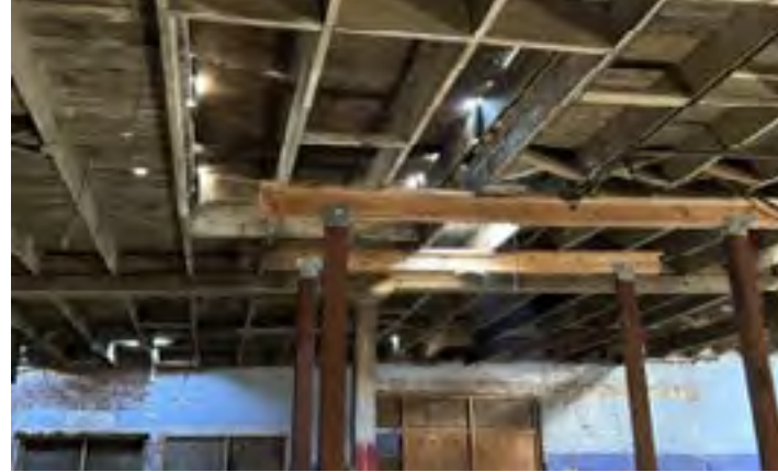
22. Damaged portion of roof with shoring.
